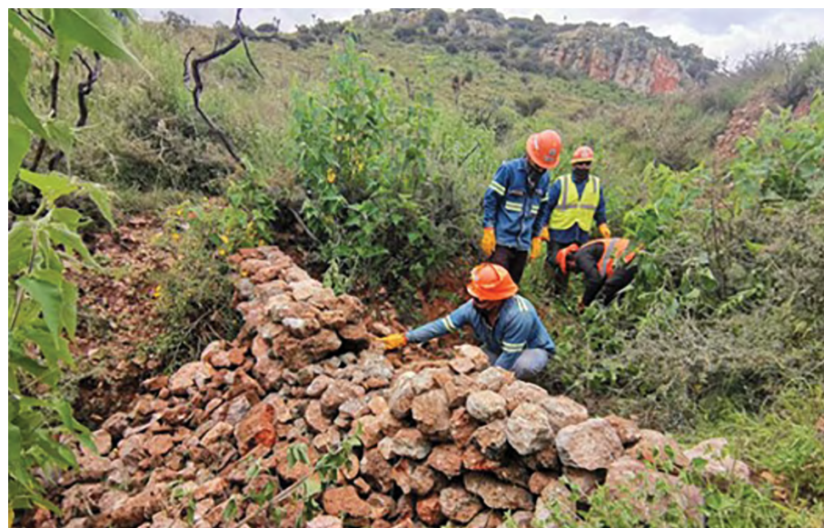
Rock terraces constructed to mitigate soil erosion as part of the soil conservation program at the Juanicipio Project.
